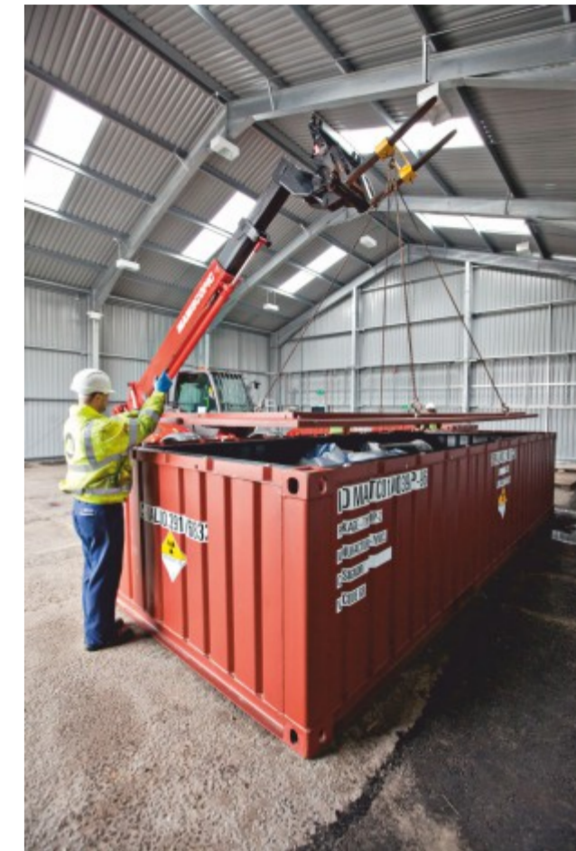
Much of the waste is low in radioactivity and can be buried safely in a series of engineered vaults being developed at the site.
